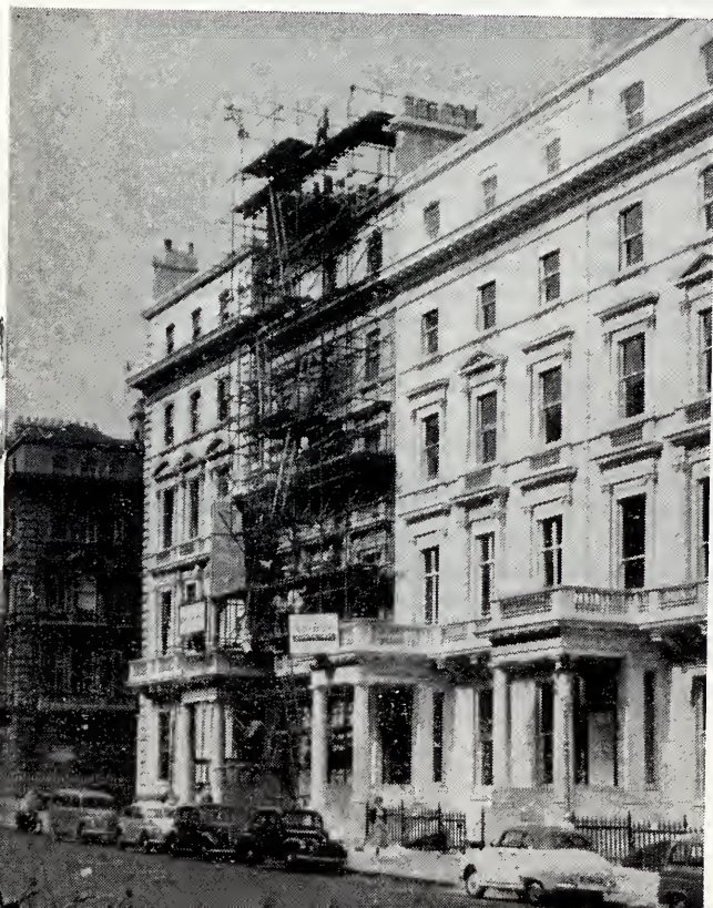
50 Prince's Gate, Exhibition Road, South Kensington, London (with scaffolding) was recently purchased by the Church. It is now undergoing extensive repairs and remodelling and will be ready for occupancy on September 1, at which time it will become the new Headquarters of the British Mission
